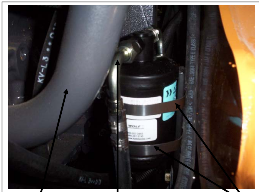
Engine oil fill pipe
